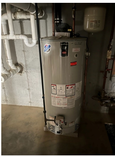
Gas Hot Water Tank
