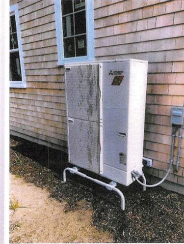
Air Source Heat Pump Exterior
