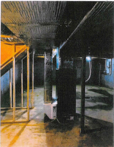
Air Source Heat Pump Interior
